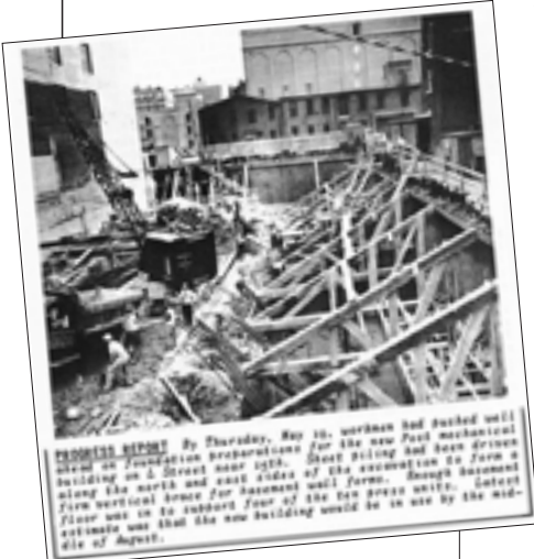
This photo of the L Street Building under construction appeared in the May 27, 1949 issue of ShopTalk.
