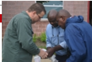
Outstanding Performance Award winners, machinist Kevin Young (left) and electrician Dwayne Jones, along with pressroom team leader Clarzell "Zell" Minor work to restore power before the ceremony and to protect electric cables from the rain.
