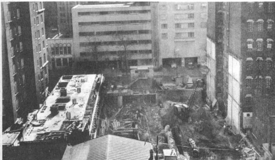
PROGRESS REPORT The Post will occupy this entire area between the Sheraton Hotel (left) and the Lenox Office Building. All foundation work is expected to be in by Jan. 1.
