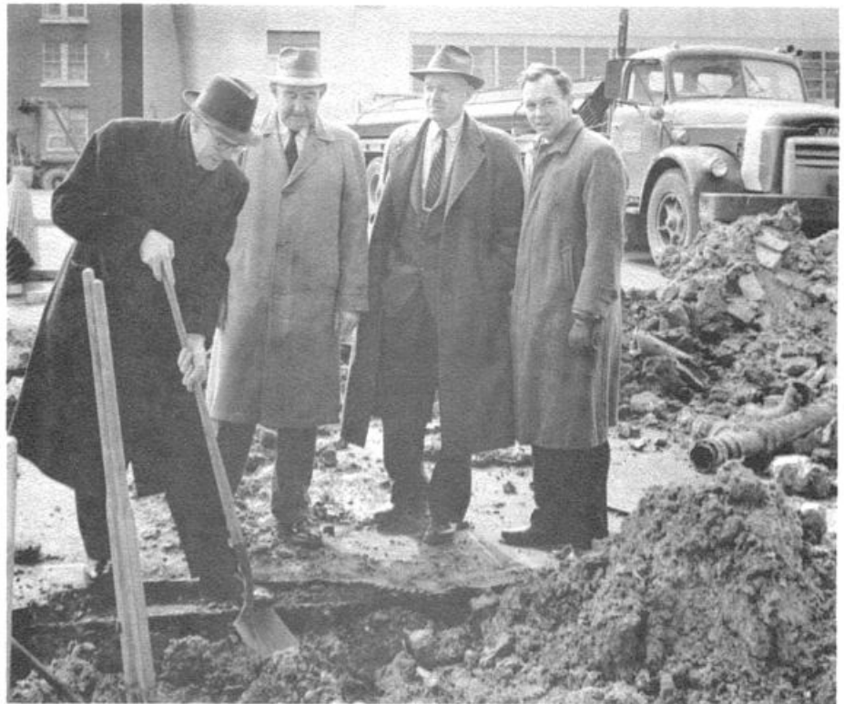
Informal ground breaking ceremonies for the Post building addition on February 16th included (left to right) John W. Sweeterman, general manager; James Gilroy, of the Albert Kahn Company; James S. Davidson Jr. of the Charles H. Thompkins Company and James P. Rogers, production engineer.
