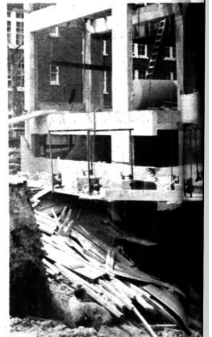
Gaping holes show area where new building off 15th Street and the stairway indicated by the will be closed in.
