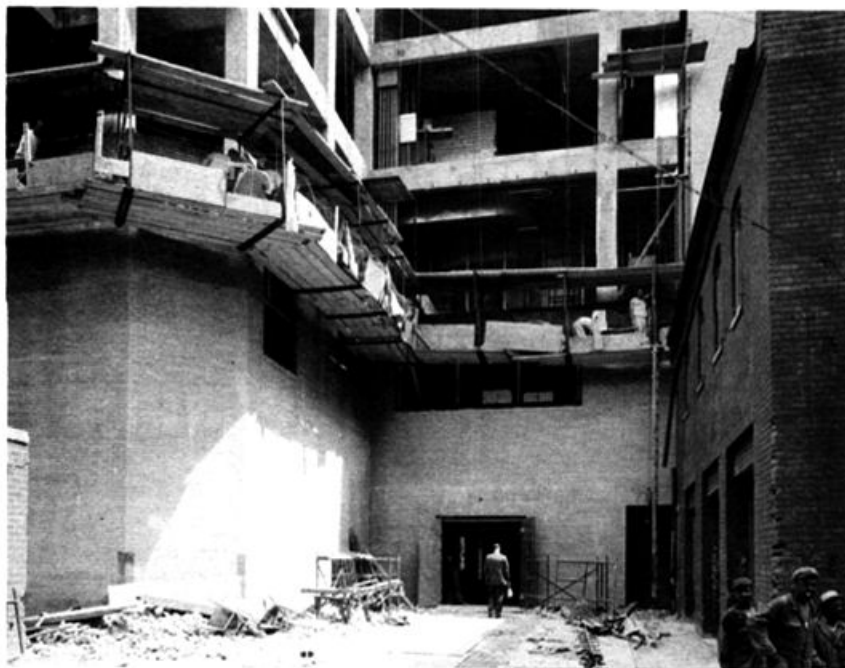
Brick masonry rises at southwest corner of building addition. This photo was taken in alley immediately behind our 16th Street Annex. Progress beyond that shown in this 2-week-old photo has been considerable.
