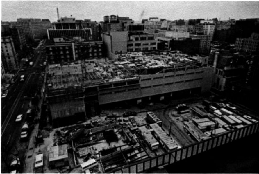
A New Year's Eve progress photo of Post building construction was taken from the corner of 15th and M streets. (Staff Photo by Matthew Lewis)
